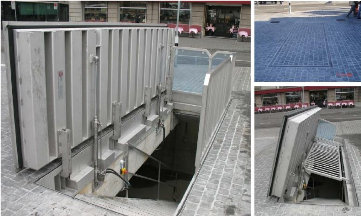
Figure 3: Floor gate at Limmatquai
