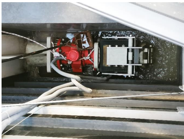
Figure 1-3 Throttle shaft with PNA integrated in the confined space.
