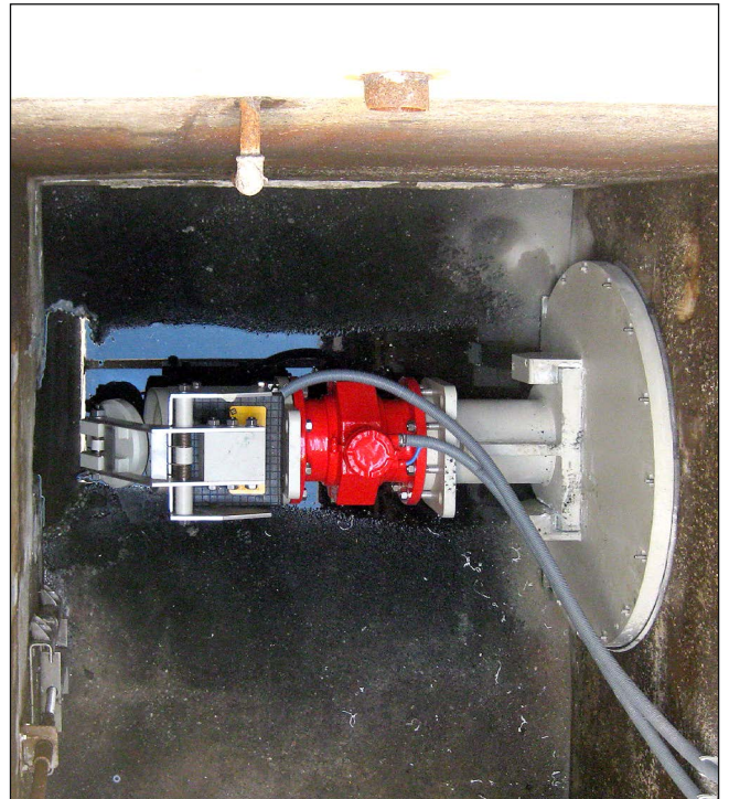
afterwards Size NW 200 pneumatic outflow control
