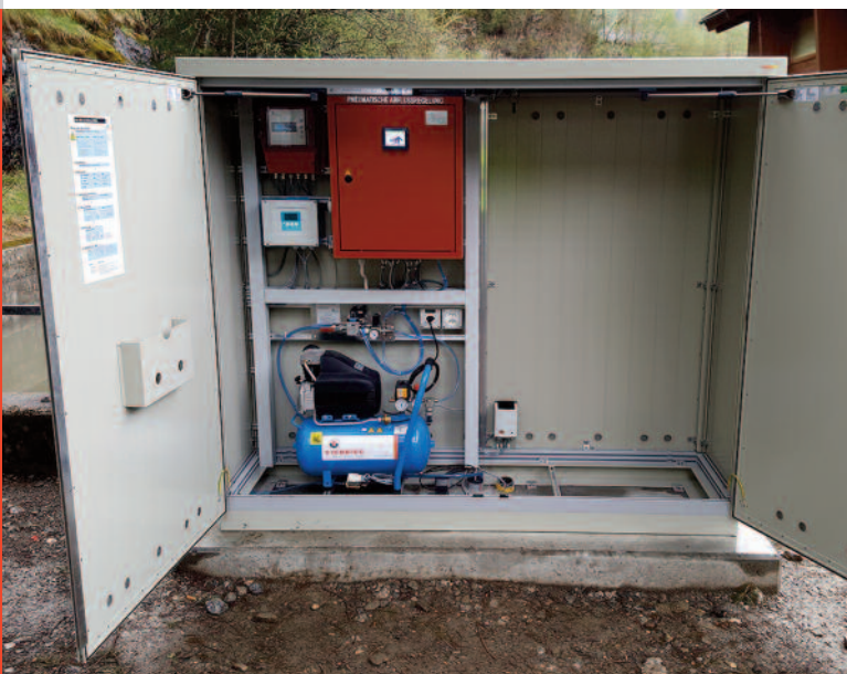
View of the booth with the control cabinet of the pneumatic outflow controller of the storm overflow basin at Galgenbühl.
