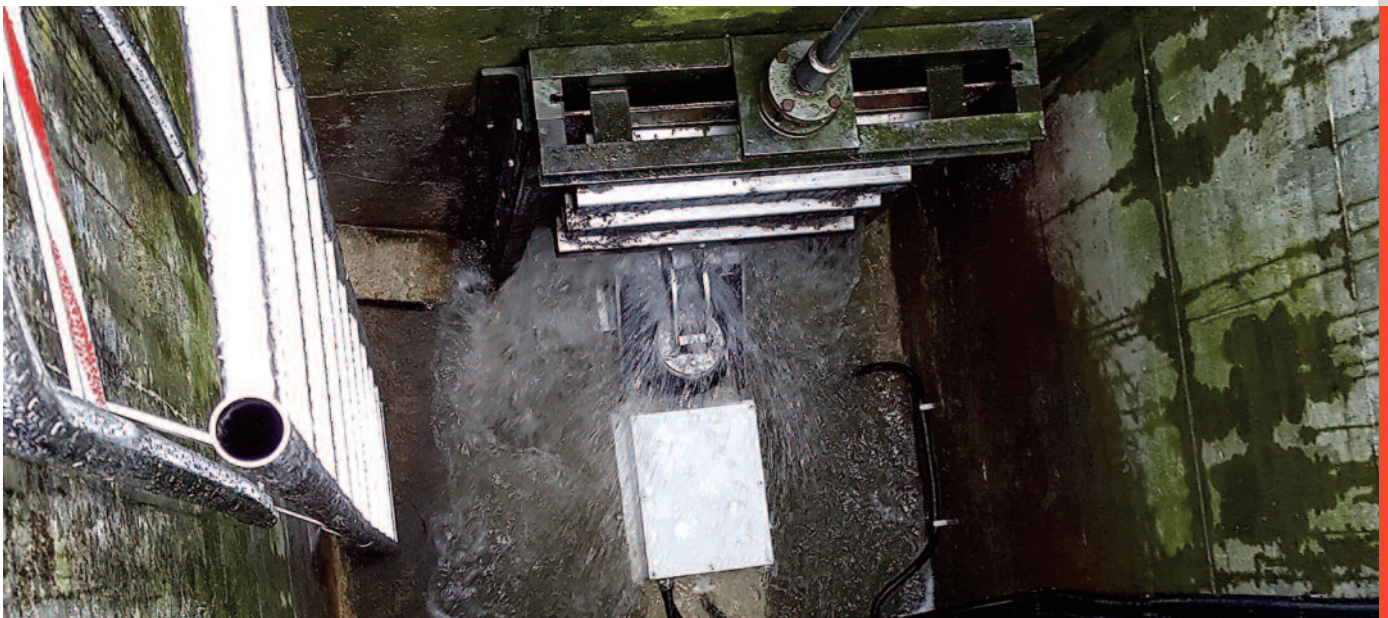
The partly filled pneumatic outflow control measures and limits the flow dynamically.
