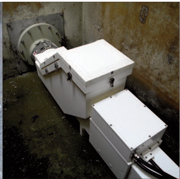
The partly filled pneumatic outflow control unit set up dry in the shaft also measures the flow.
