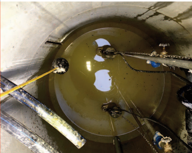
The well of the main pumping station, the only station with two pumps that operate alternately.
