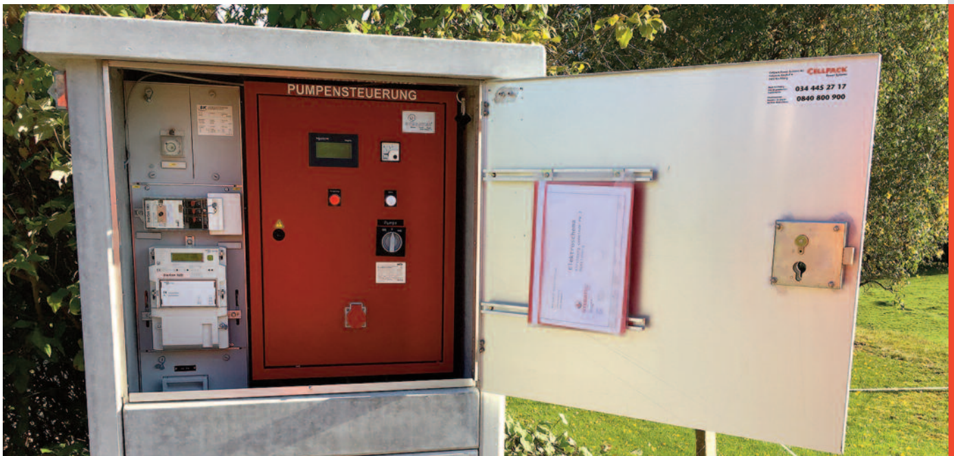
View of one of the new booths with the compact pump control (right) and the energy meter (left).
