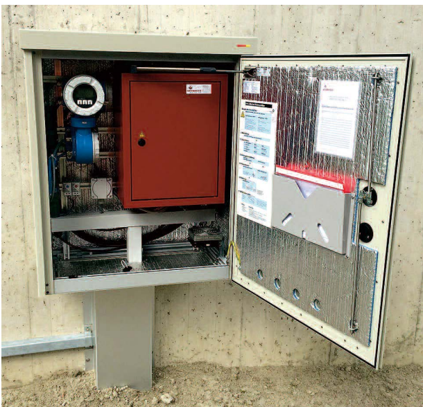
View of the control cabinet of the measuring station in Raron.
