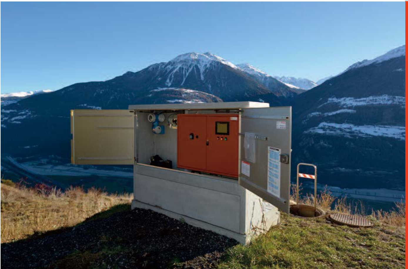
The control cabinet of the Erschmatt (Leuk municipality) storm-water basin is located prominently high above the main valley.
