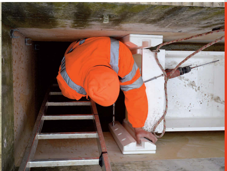
Installation of the part-filled stationary flow measurement in the outlet canal of the Radet waste water treatment plant.
