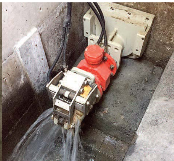
Eischoll measuring station: MID-controlled pneumatic outflow control.
