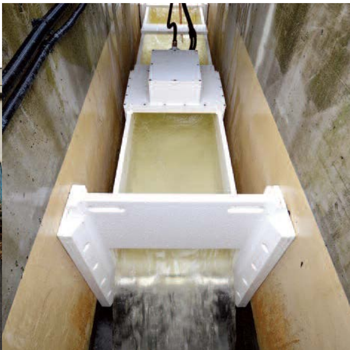
The outflow from the Radet ARA is now measured by a part-filled stationary flow measurement system.
