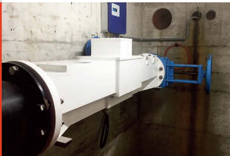
Oberems measuring station with part-filled stationary flow measurement.
