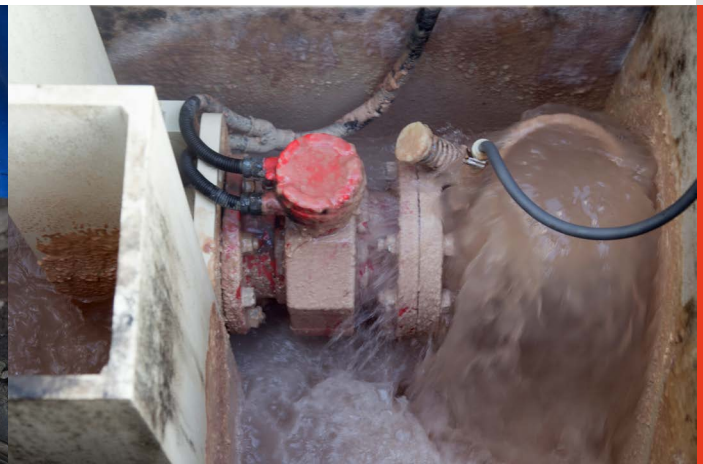
The waste water flows through the flow meter. The water samples are transferred into the collecting vessel by the hose.
