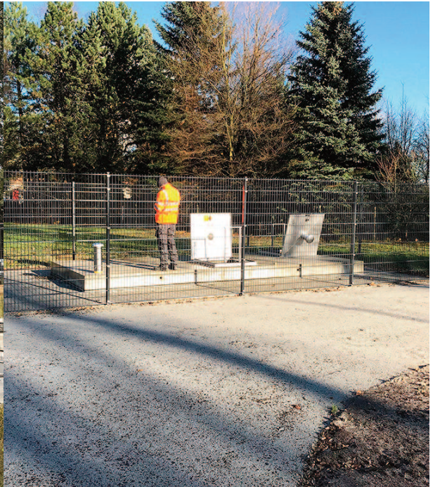
The finished shaft with a fence around it and the open hatches for maintenance and inspection.
