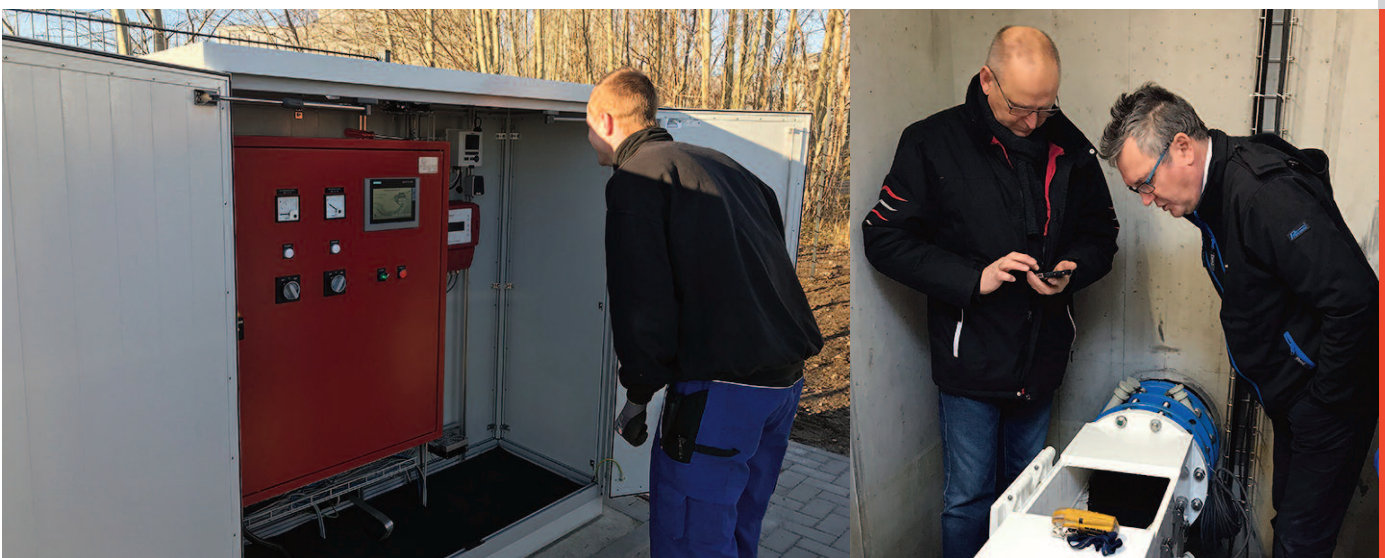
The control cabinet of the North metering pipe of size DN 300. The two measuring transducers are seen on the right of the control cabinet.
