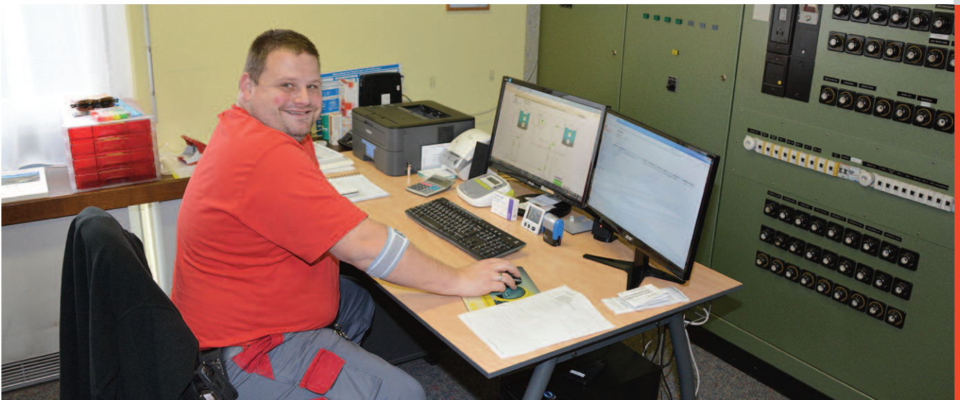
Official in charge Michel Hess at the sewage treatment plant "Am Twannbach" controls all processes with ARAbella online in the cloud.
