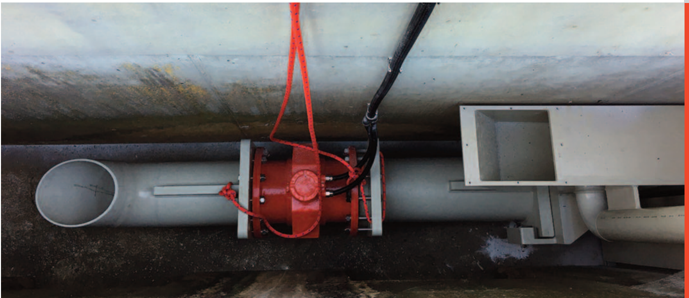
Installation of the IDM unit of the stationary flow metering system and of the impoundment pipe in one of the two shafts.
