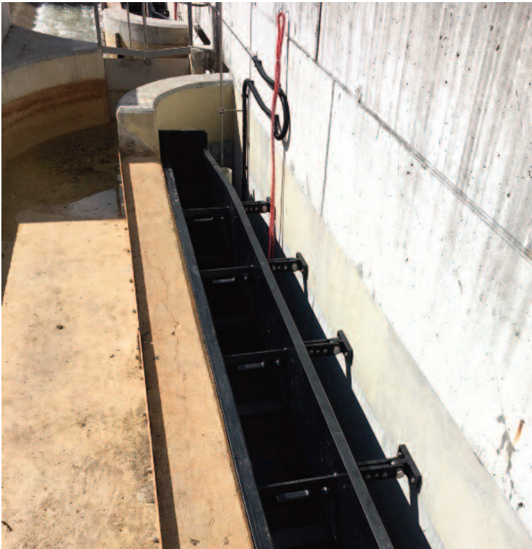
View into the right, dry outflow channel downstream the preliminary sedimentation section.
