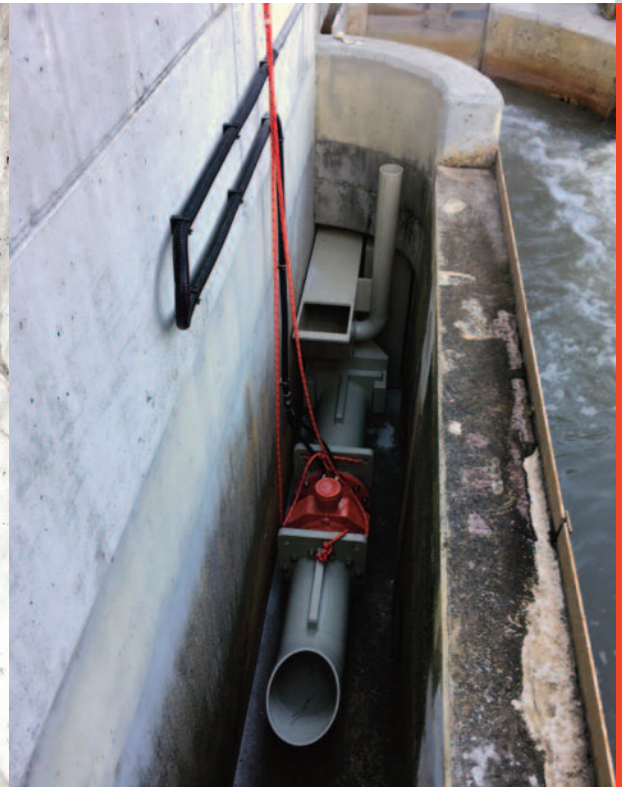
The left channel during the installation of the IDM measuring unit. High water flows over the edge that is running from the right lower edge upward in the picture.
