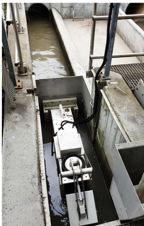
Figure 1: Installed inlet control
