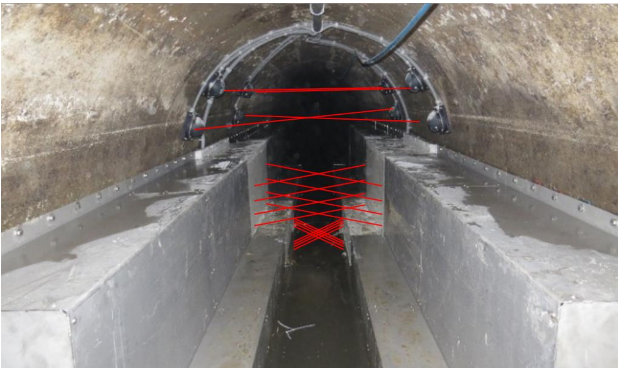
Figures 2 + 3: Flow measurement in the DN 2000 storage sewer with inserted dry weather channel for the large measuring range of 50 - 2000 l/s. In the bottom picture, the red lines depict the ultrasonic measuring tracks.
