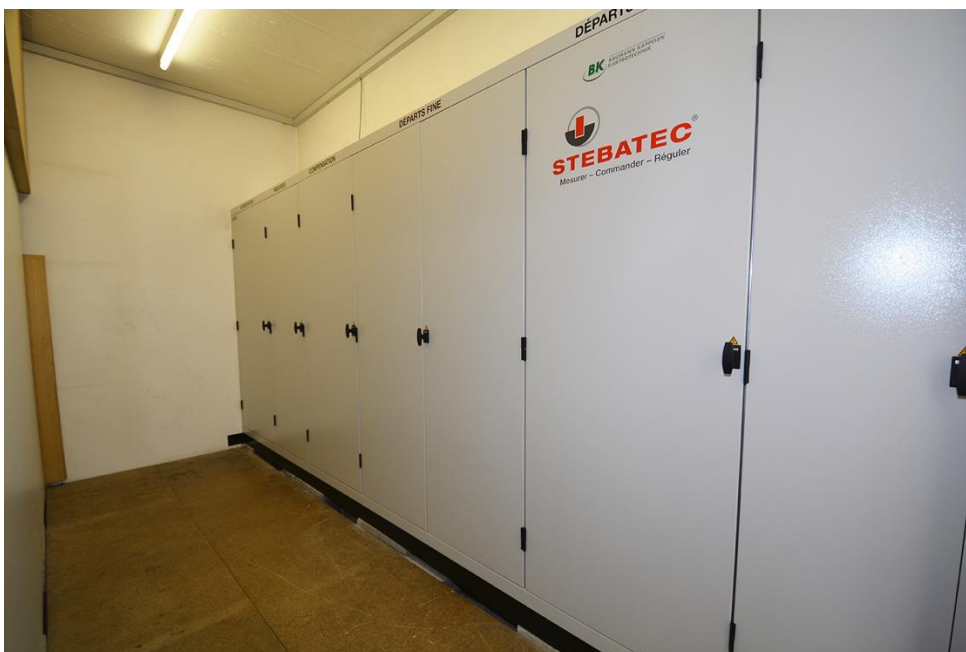
The new switchgear cabinets with the modern electrical distribution once again.
