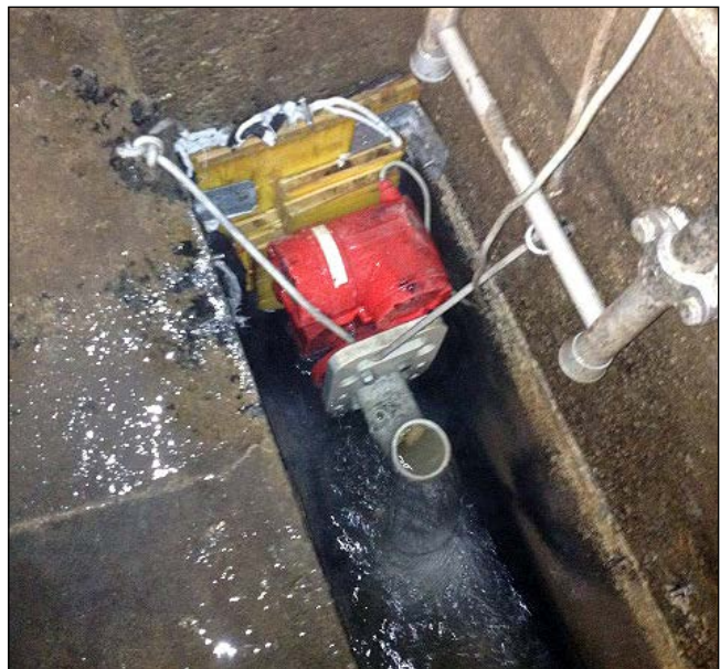
Walliswil b. B., Pumpwerk – DN 150
