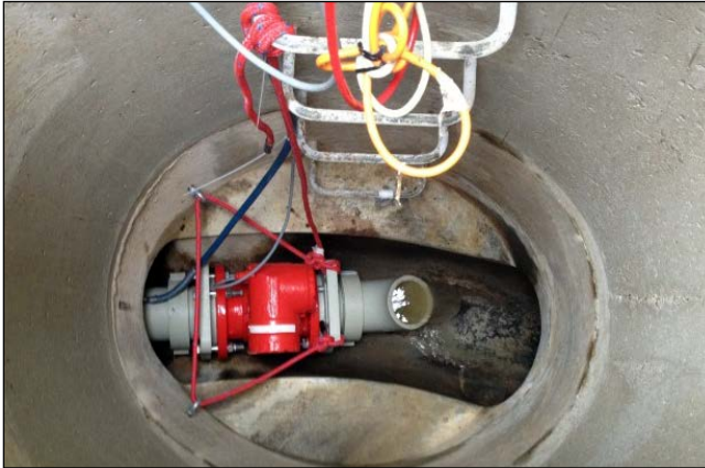
Walliswil b. W., Pumpwerk – DN 150
